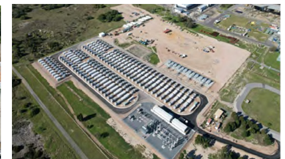
Torrens, Australia – 1.2 GWh Project
