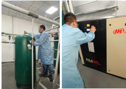
On site handling of abnormal pressure vessels in the air compressor room of the factory in Xiangcheng
